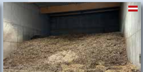
Biomass heating plant - Austria
