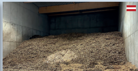
Biomass heating plant - Austria
